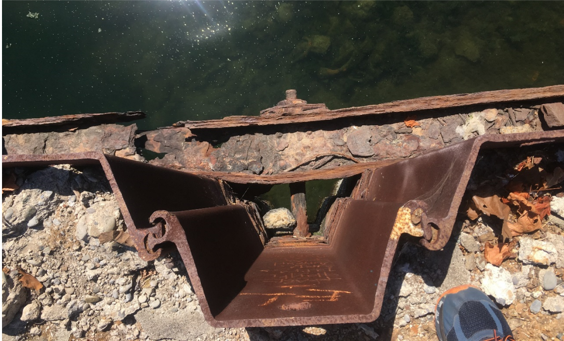
Figure 3: Damaged waler and anchor rod
