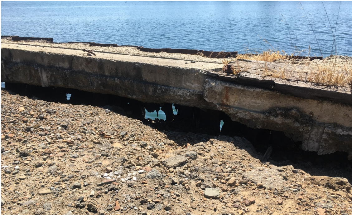
Figure 4: Corroded sheet-pile wall and ground subsidence
