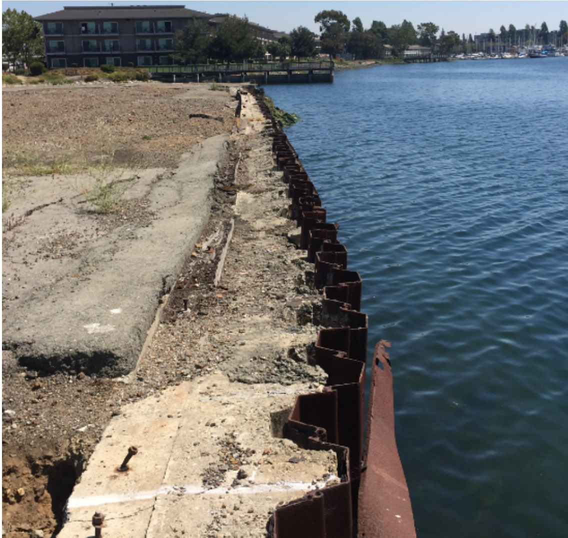
Figure 2: Existing bulkhead bowing and showing deformation
